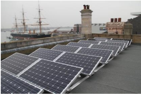
Built-Added Photovoltaics (BAPV)
